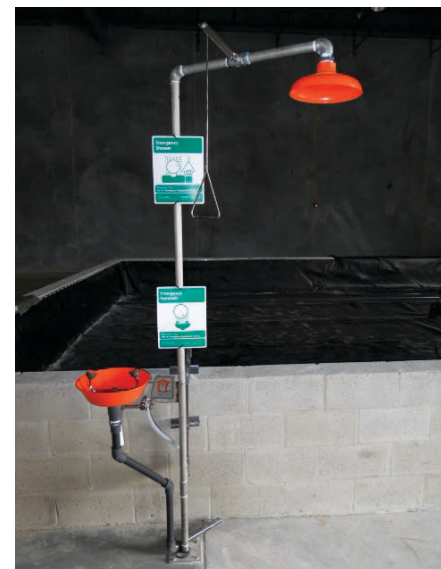
EMERGENCY EYE WASH & SHOWER
